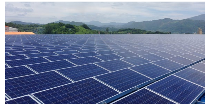
Korea Energy Power Plant
